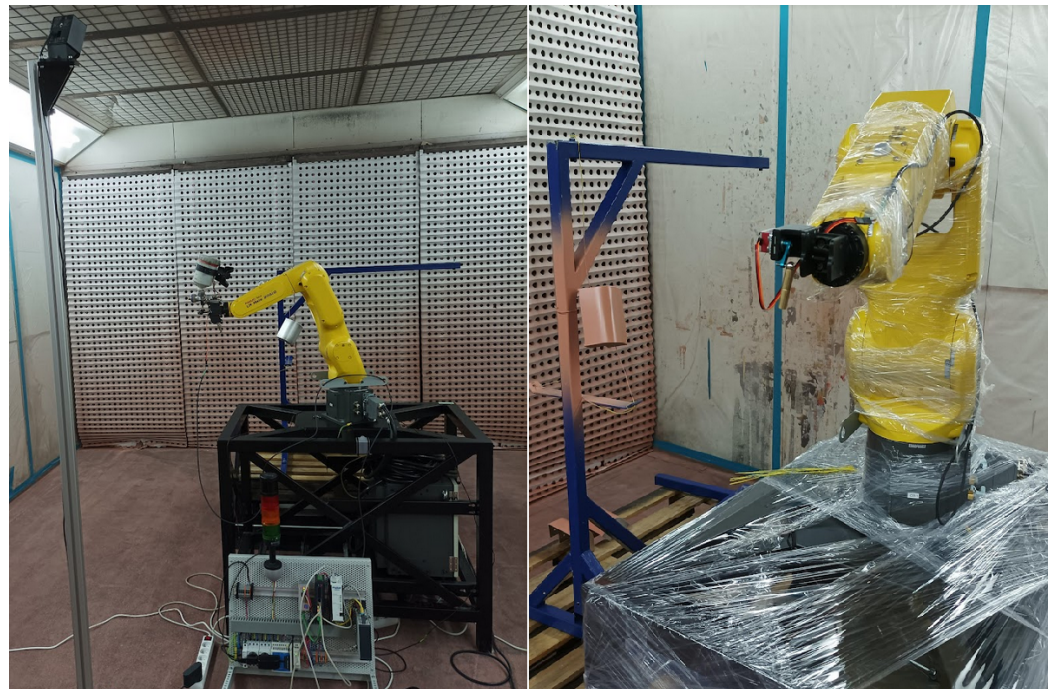
Figure 14. Pilot application—flexible spray coating robotic cell, (left) Fanuc LRMate 200iD robotic arm equipped with the tracking system, (right) detailed view.
