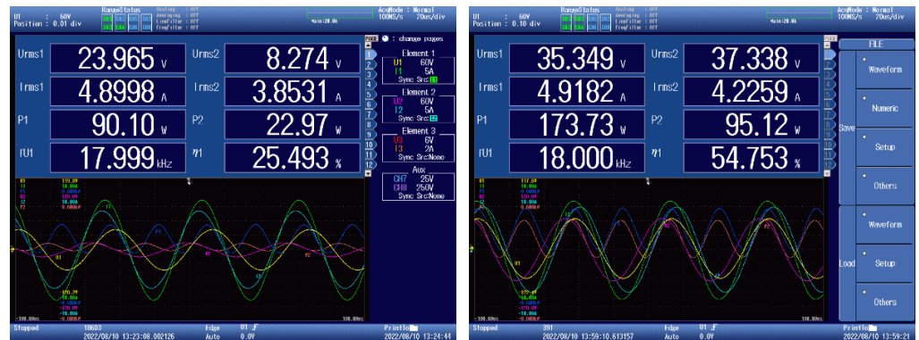
Figure 7. System quantities measured for 2 Ω (left) and 4 Ω (right) of load connected to the secondary voltage.
