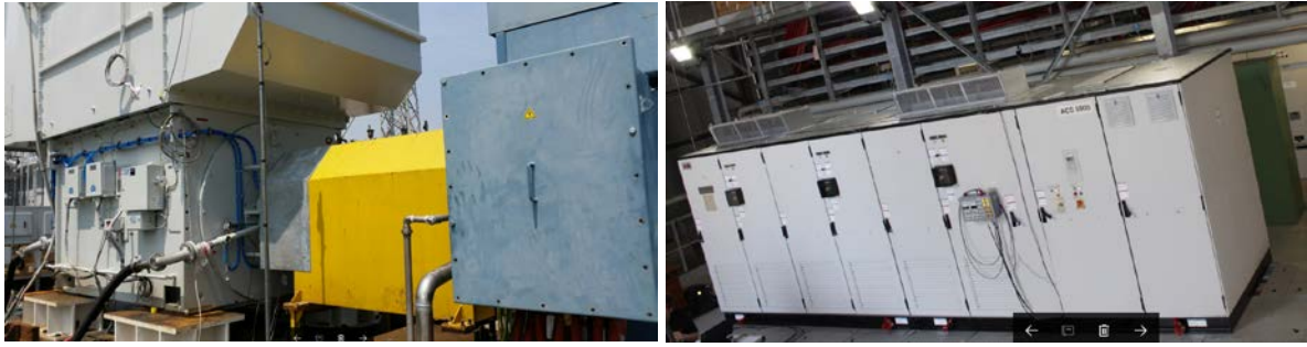
Figure 8-10: Full load combined test of drive system as per Table 16
