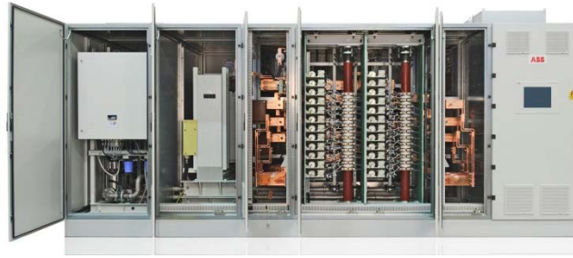
Figure 8-5: LCI converter with open doors (courtesy of ABB)
