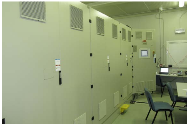
Figure 8-2: LCI drive inside container of drive system as per Table 8 (courtesy of ABB)
