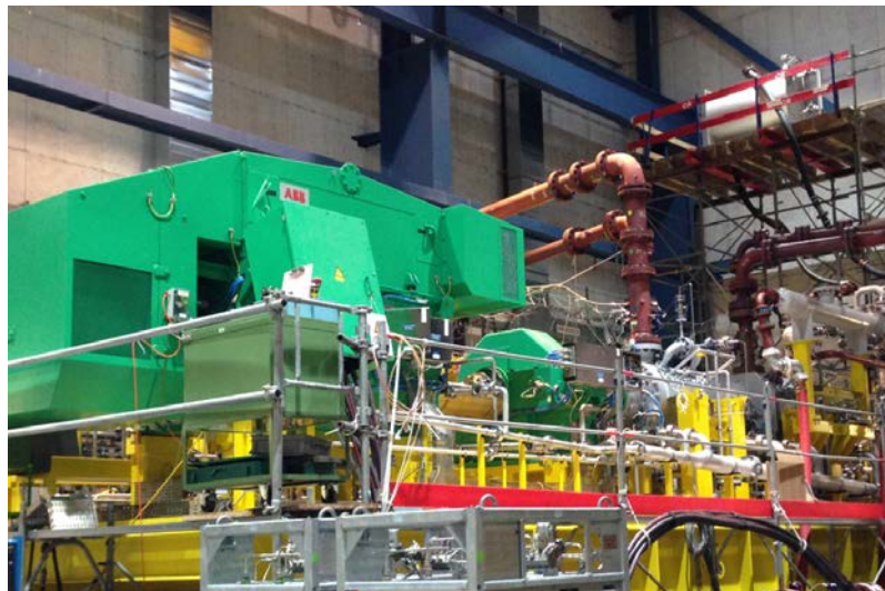
Figure 8-12: String test of drive system as per Table 19 (courtesy of ABB)
