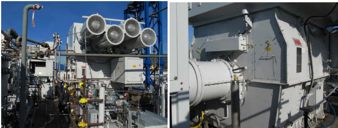
Figure 8-1: String test of drive system as per Table 7 (courtesy of ABB)
